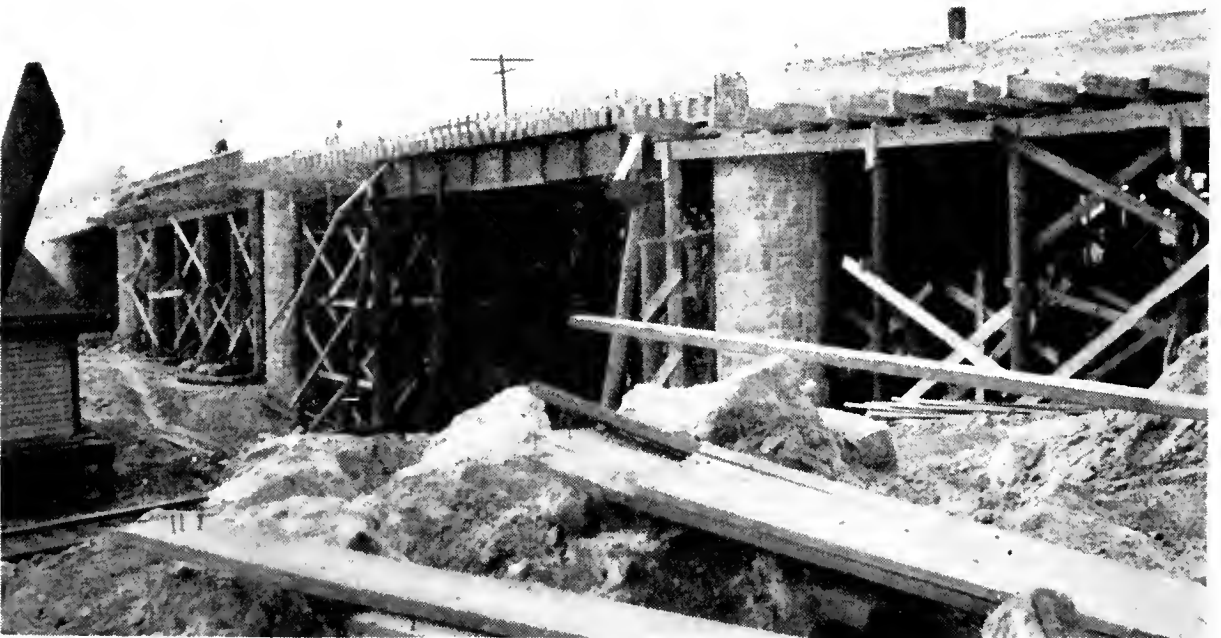
BRIDGE OVER WESTERN MARYLAND RAILROAD TRACKS, MD. ROUTE 128 AT GLYNDON, BALTIMORE COUNTY. UNDER CONSTRUCTION JUNE 30, 1948
